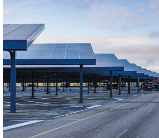
One of the largest European solar canopy plants is under development at Disneyland Paris, to be completed in 2023.
